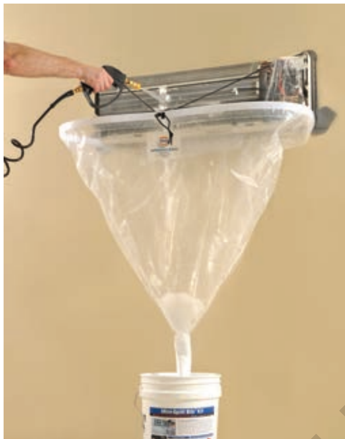
Figure 23-64. Use a pressurized washer with a plastic bib and bucket while cleaning an indoor unit's evaporator.
