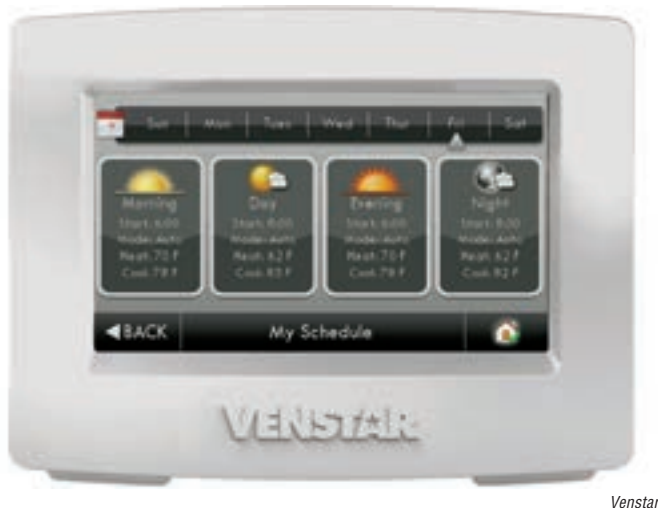
Figure 23-13. This programmable thermostat's display is showing the time and temperatures for system operation for Fridays.
