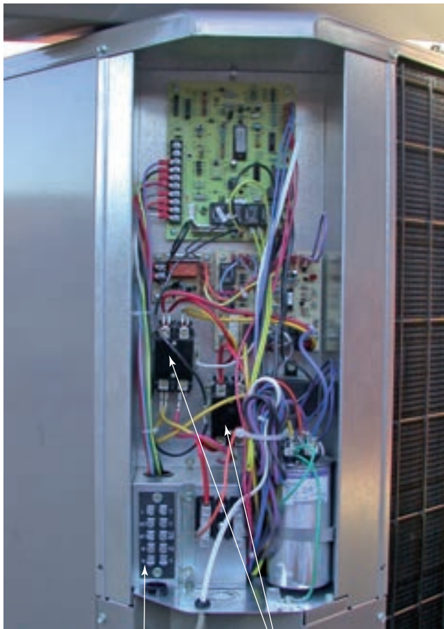
Thermostat control wiring terminals
