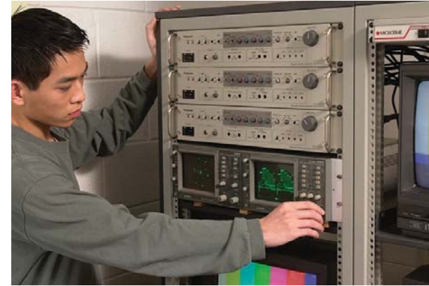
Figure 2-6. The video engineer uses specialized test equipment to examine and maintain consistent picture quality.
